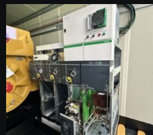
Cellules haute tension
